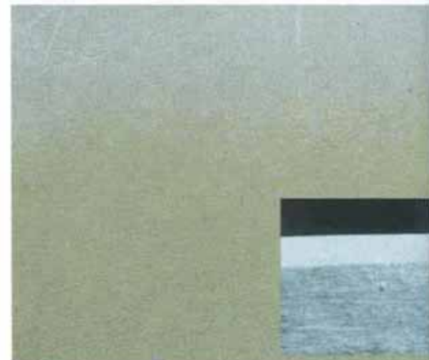
24 - Yellowing caused by thick gel coat (inset shows 55 mil thickness of white gel coat)
