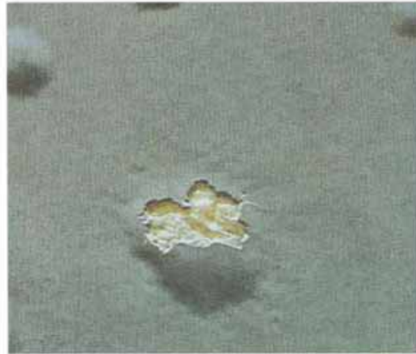
4 - Blisters - caused by catalyst drop
