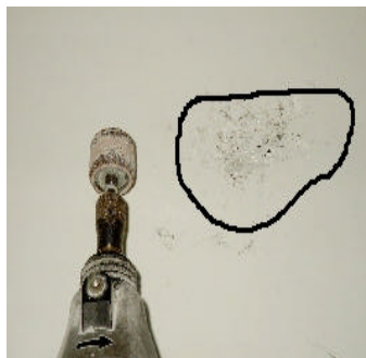
Figure 9 Defined Area of Damage
