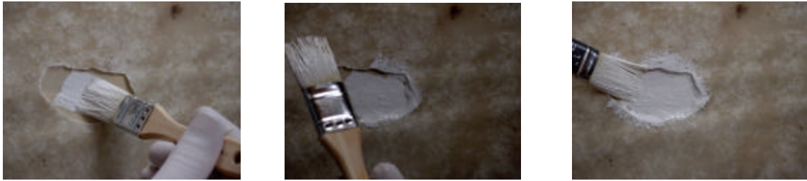
Figure 19, 20 & 21 I use a disposable brush to apply the gelcoat to the project.
