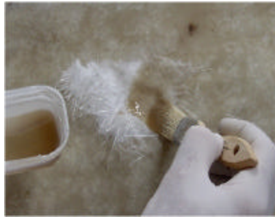
Figure 23 saturating the mat
